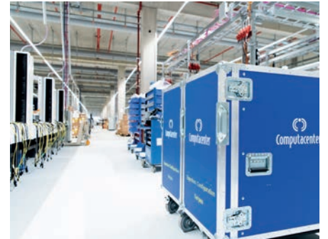
Data center and network deployment
